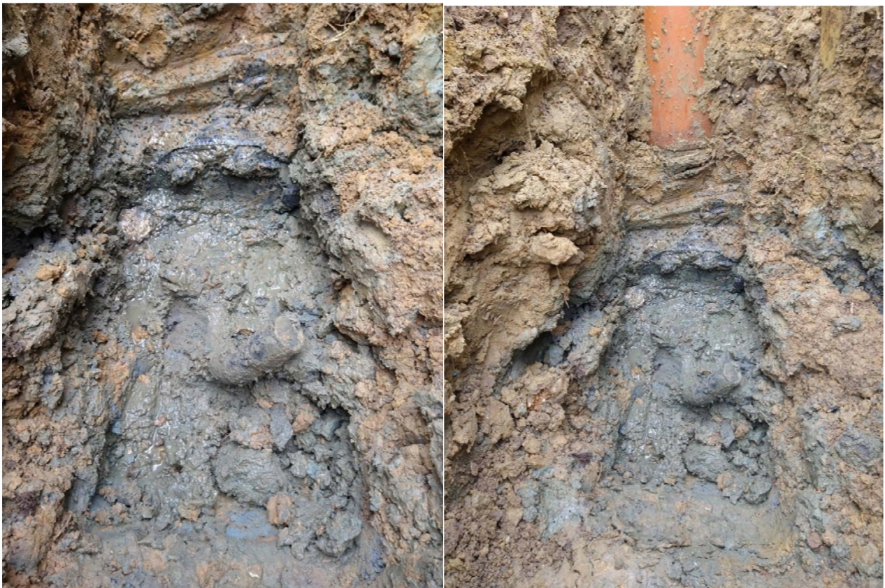
Photo 1. Gas Main Trench – Indicating groundwater seepage at 0.8mBGL and heavy clay soil.
