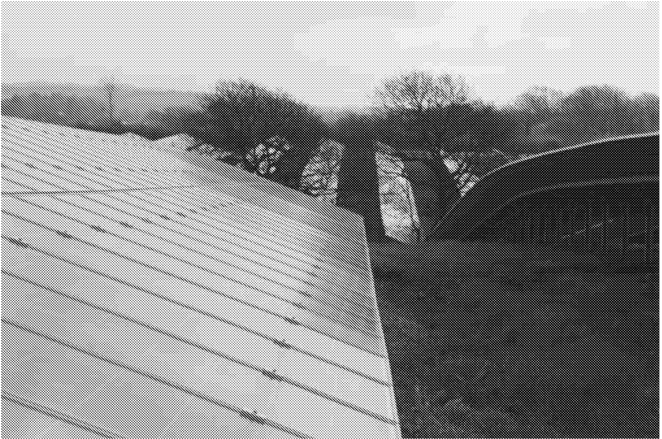
Figure 3: Example of solar panels following topography at Jordanstone Solar Park
