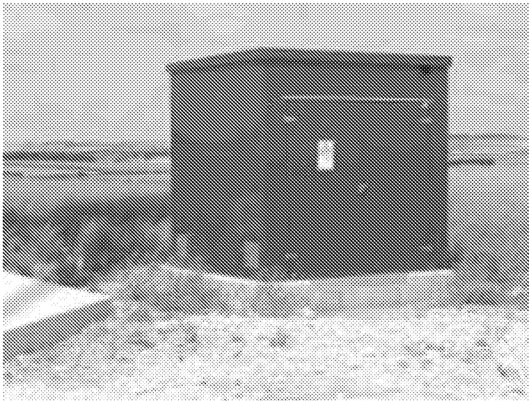
Figure 1: Example GRP Substation
