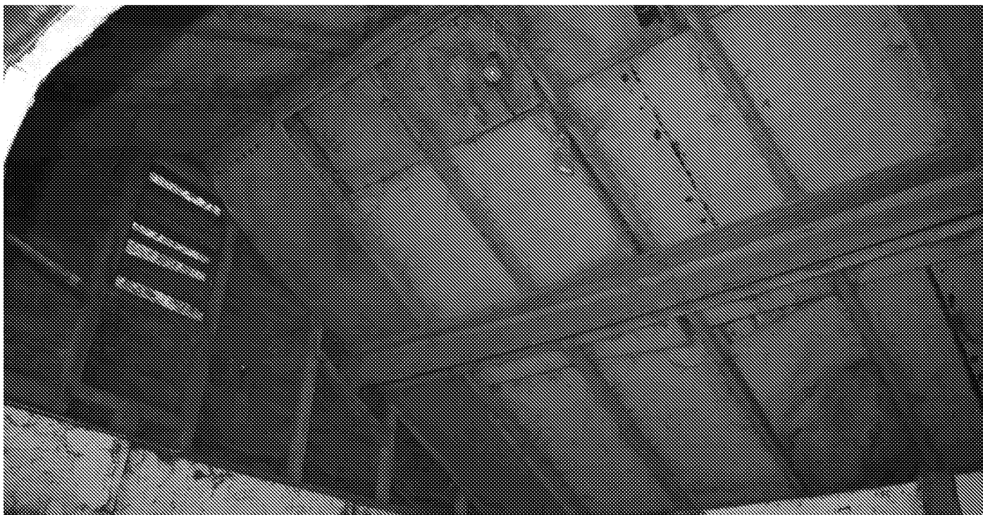
Photograph No. 09 - Building 2 - No loft cavity and tightly sealed panels against the rafters.
