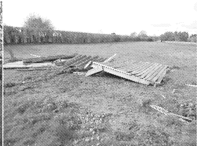
TN1: Demolished outbuilding remains in northern parcel of land.
