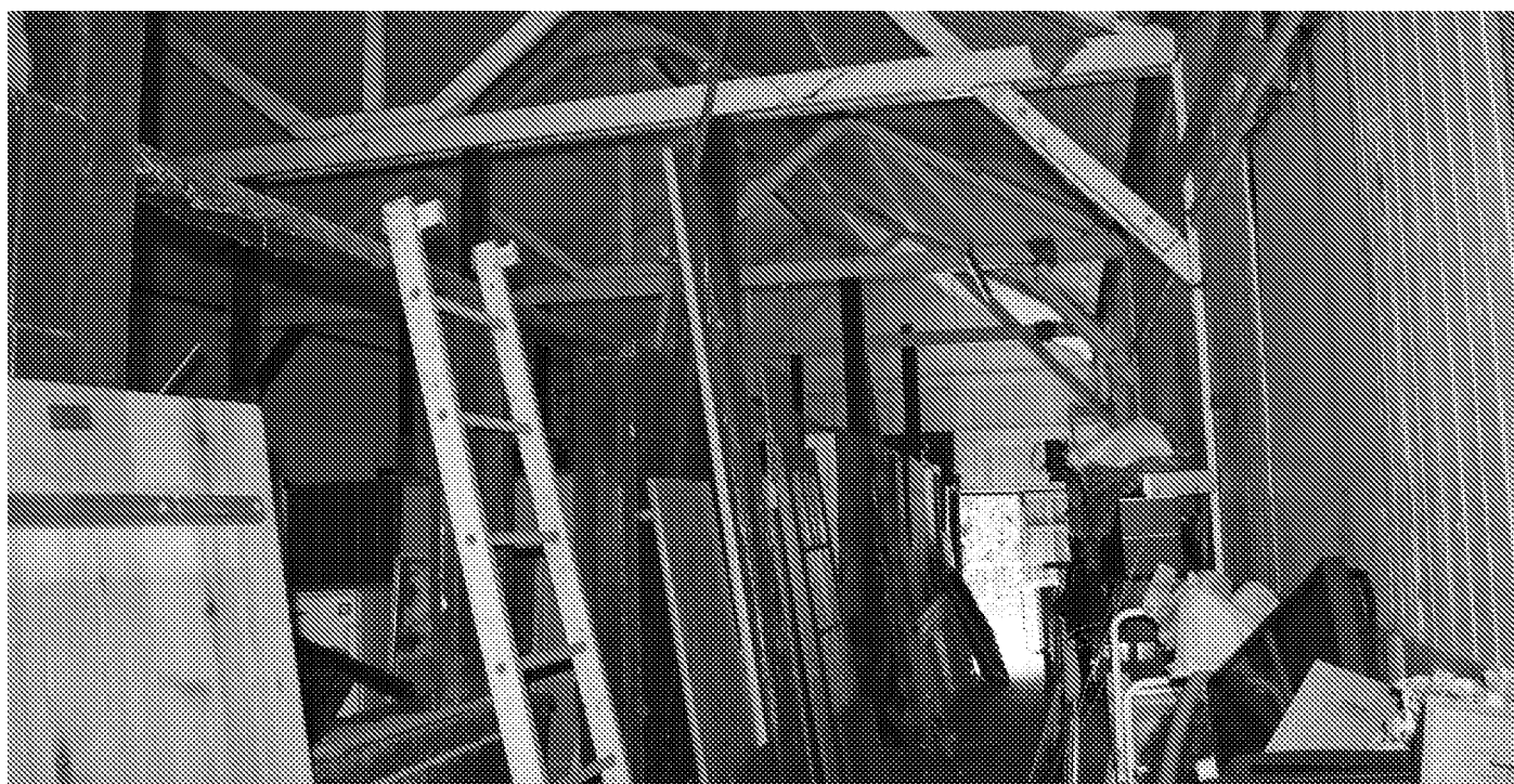
Photograph No. 06 - Building 1, internal view of section 2, rafters sealed to wooden panneling.
