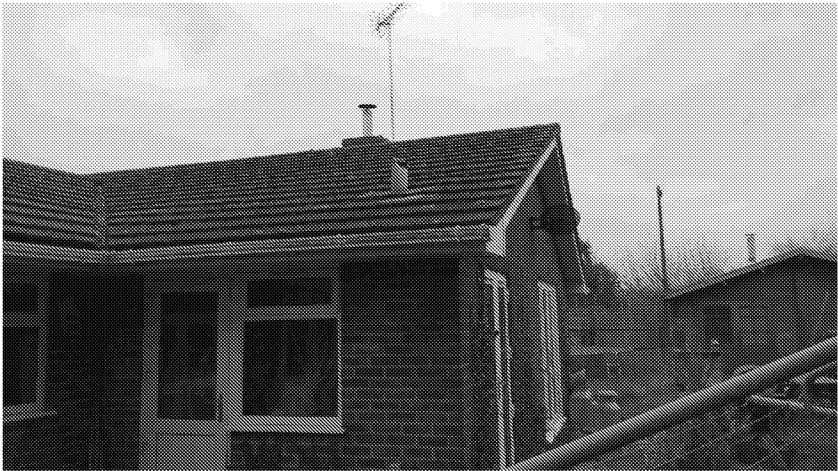
Photo 8. Roosting feature in the form of gap in the tiling beneath the flashing surrounding the base of the steam vent on the southern side of the property.
