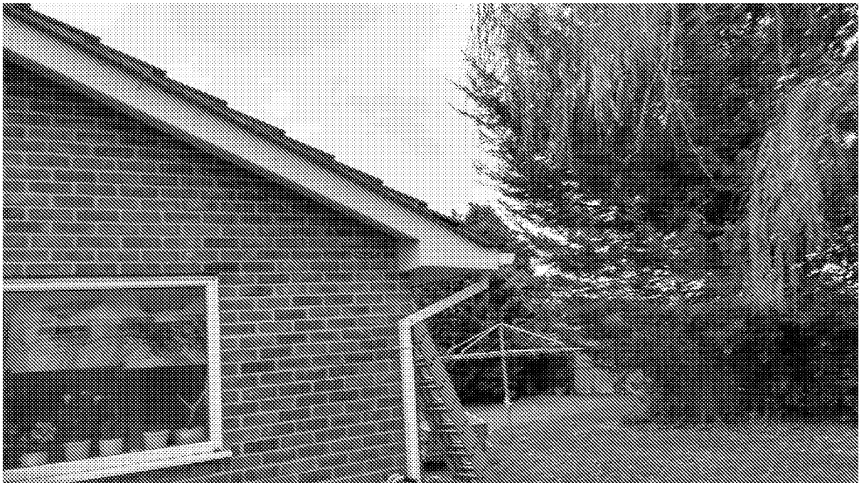
Photo 7. Roosting feature in the form of a gap between the tiling and the brick work at the western gable end of the property.
