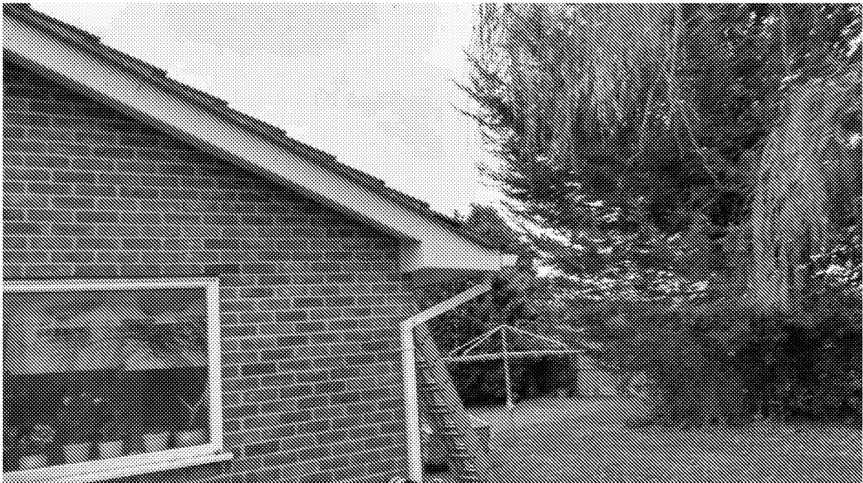
Photo 8. Roosting feature in the form of a gap between the tiling and the brick work at the western gable end of the property.
