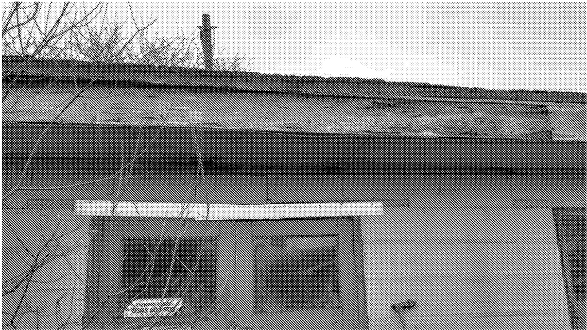
Photo 7. Roosting feature in the form of a gap present within hollow wooden facade on the northern side of building 3
