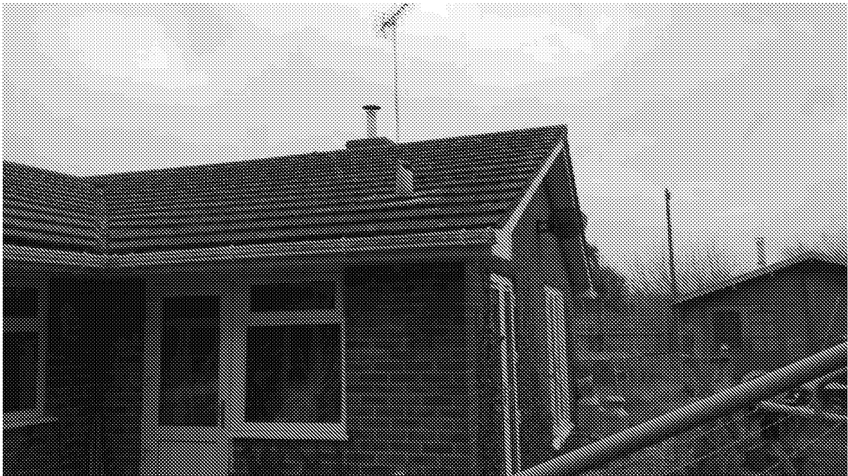
Photo 9. Roosting feature in the form of gap in the tiling beneath the flashing surrounding the base of the steam vent on the southern side of the property.
