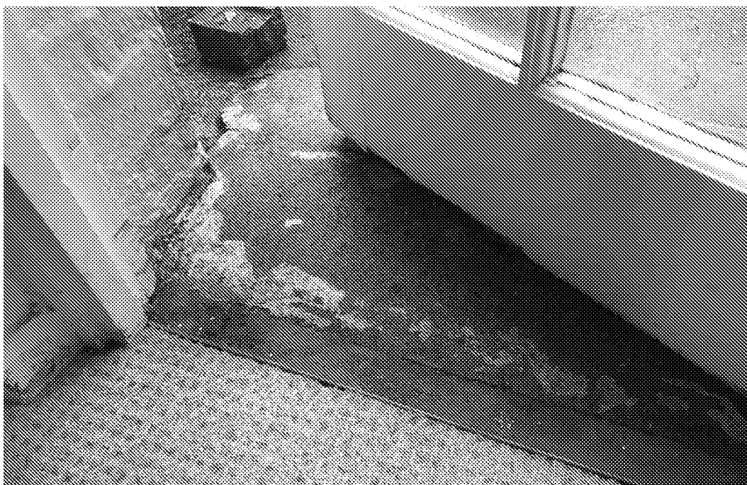
Figure 3 - Existing door lack of sill and rot
