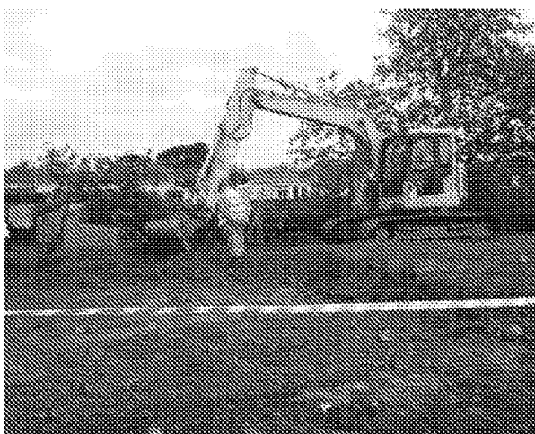
Investigation to find extent of AIB
