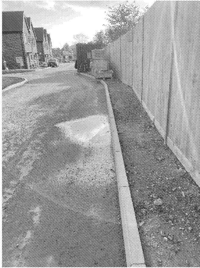
Figure 26: Photograph of Proposed Position of Gully
