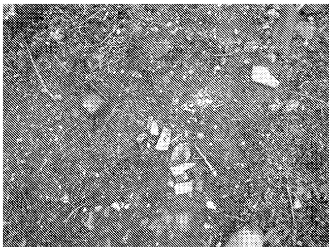
Plate 9: Fragments of asbestos cement were also noted scattered across the site surface.
