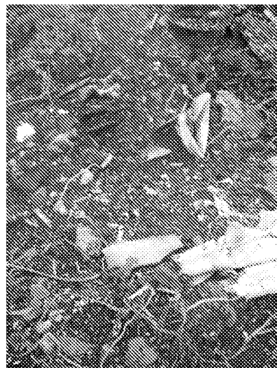
Plate 8: Fragments of asbestos cement were noted on the surface of the stockpile.
