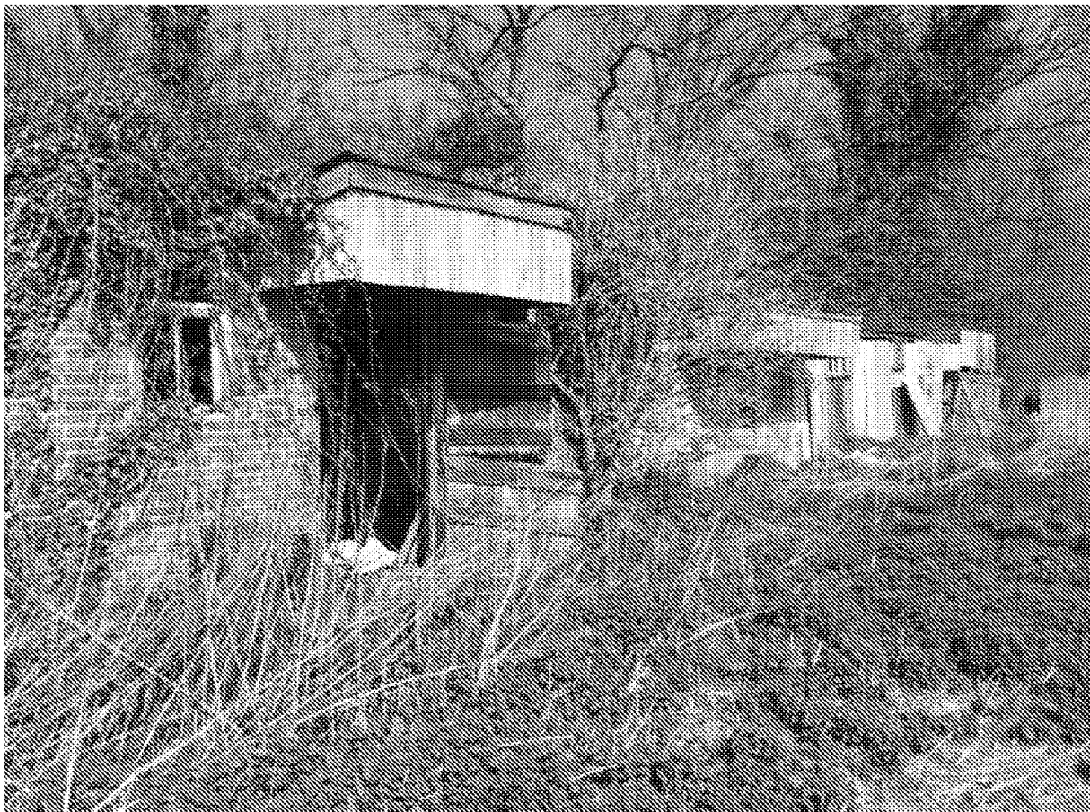
Figure 10. View of the dilapidated brick and single skinned walled shed with corrugated chrysotile roof from the south.
