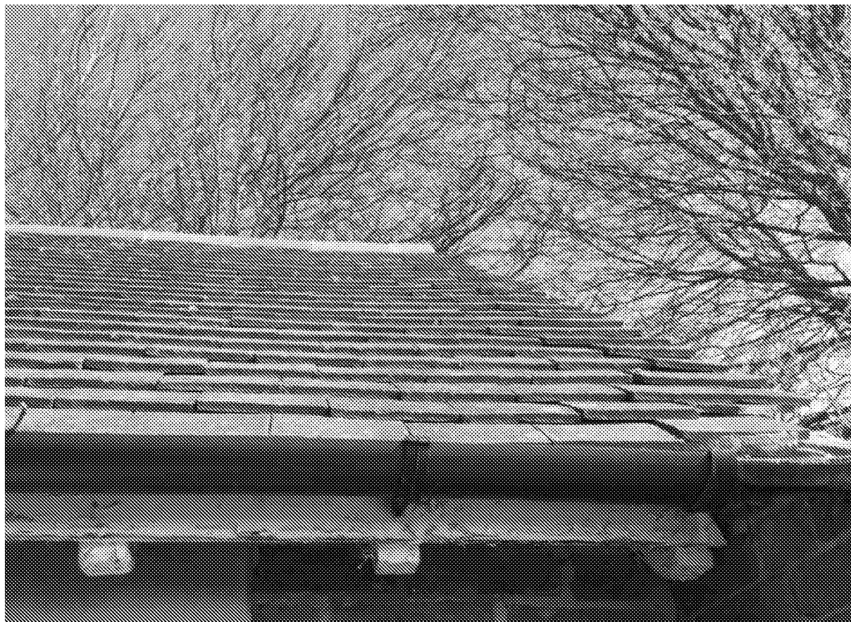
Figure 18. Lifted tiles with the potential to support bats on the southern face.
