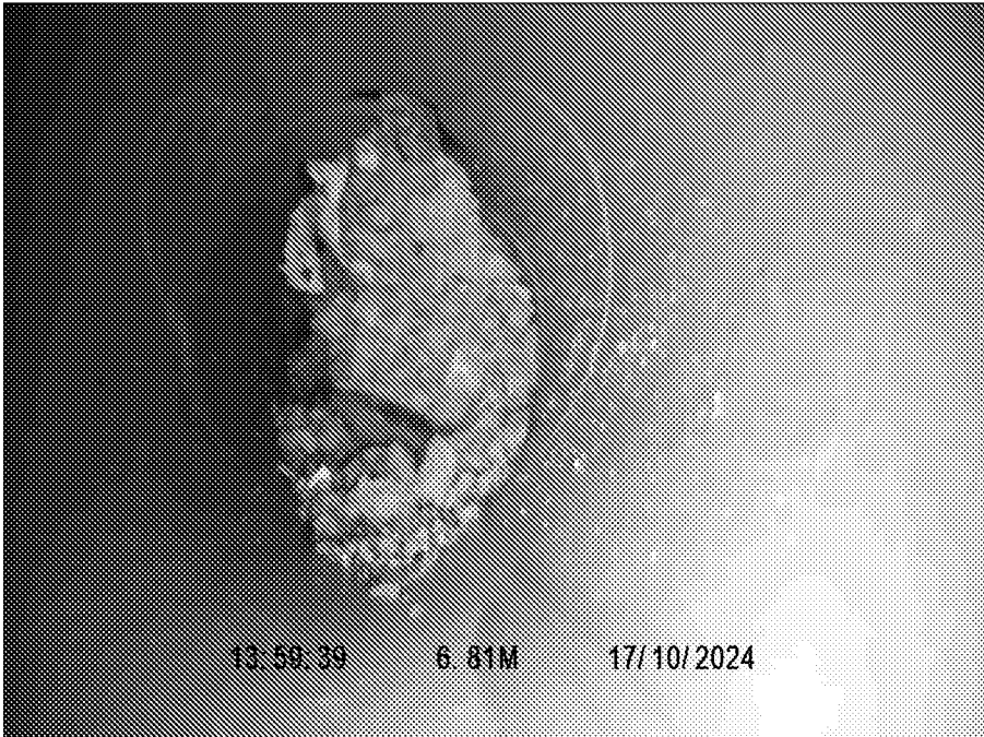
S63X_7efb1fa8-a72f-4fc9-89ee-02cd8aeeef017_20241026_135335_494.jpg, 00:00:25, 6.81 m Cracks, multiple from 12 o'clock to 11 o'clock
