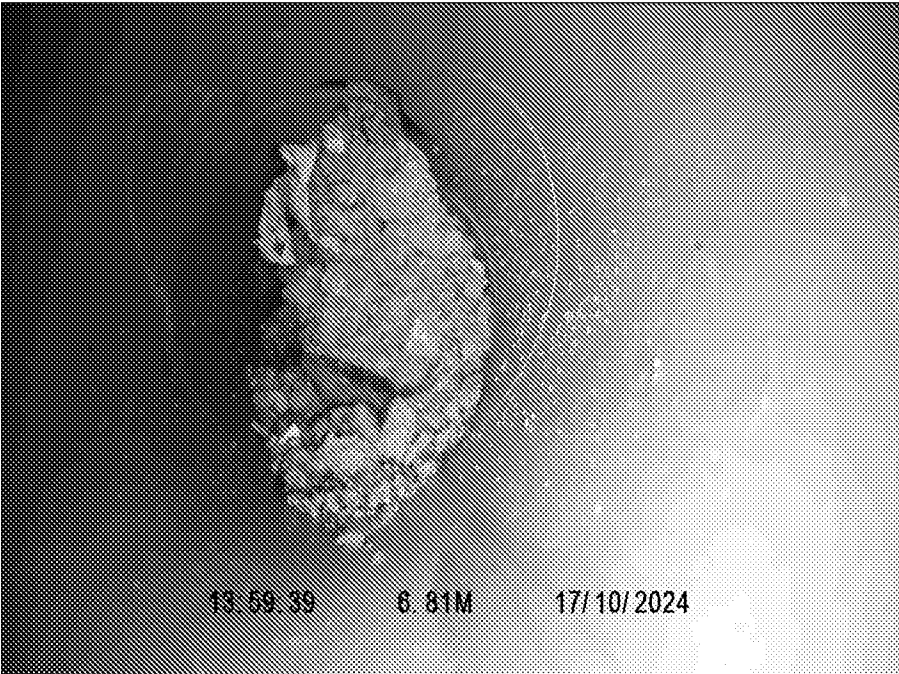
S63X_54743745-6956-4ae3-92c5-5050ab27cf3e_20241026_135333_545.jpg, 00:00:25, 6.81 m Collapsed drain or sewer
