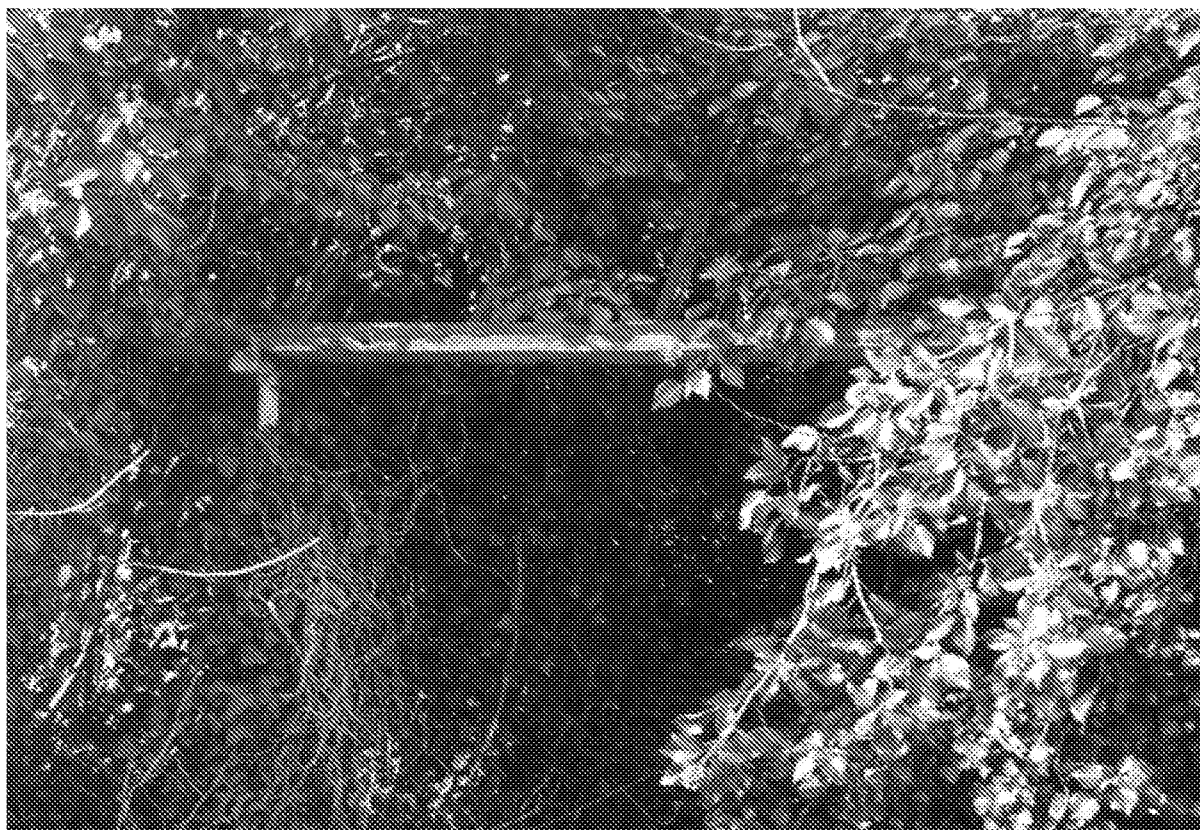
Figure 15. Derelict shed structure completely covered by ivy.
