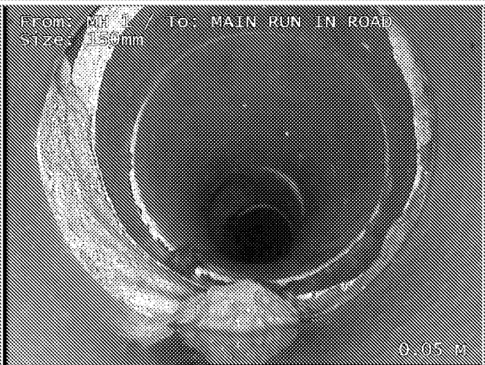
Joint displaced 20mm
