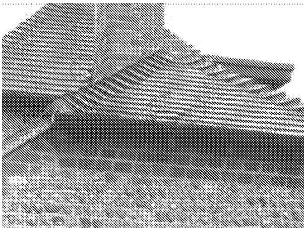
Raised tiles on north elevation
