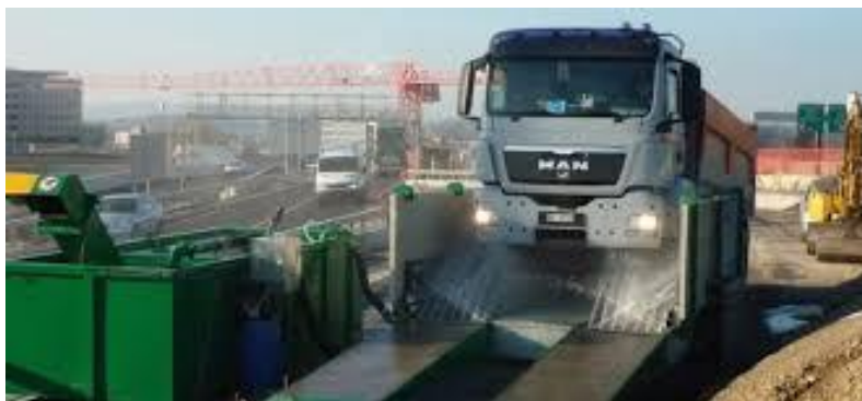
Example wheel washing facility
