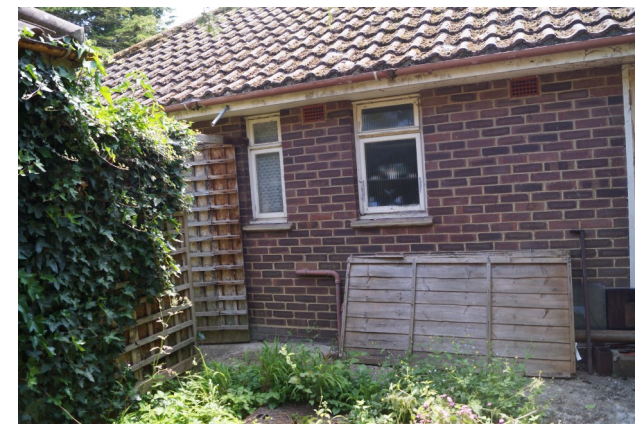
Windows at Nyasa facing boundary
