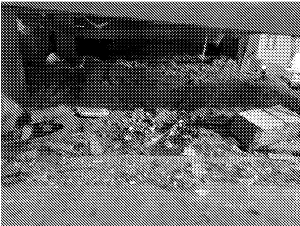
Stairs laid on mud:
