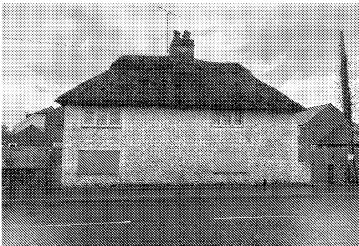
Fig A12 - Wayside Cottage from Burndell Road, north-east elevation. This shows the thatch and block ridge design. The poor condition of the thatch is clearly visible from the road as are the rotten and broken casement windows.
