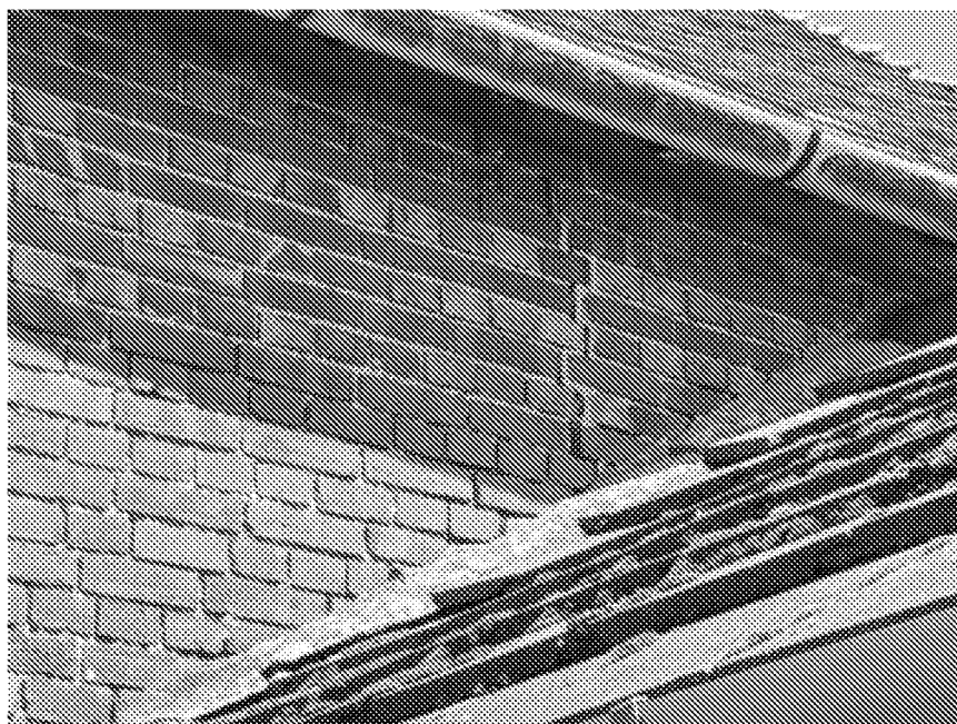
Building 2 – Side elevation showing vertical cracking in side wall abutting Building 3
