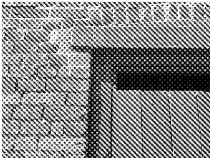
Building 2 – Front elevation showing vertical crack through the lintel above one of the doors
