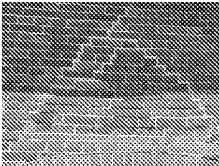
Building 2 – front elevation showing diagonal cracking above one of the doors, which has been repointed
