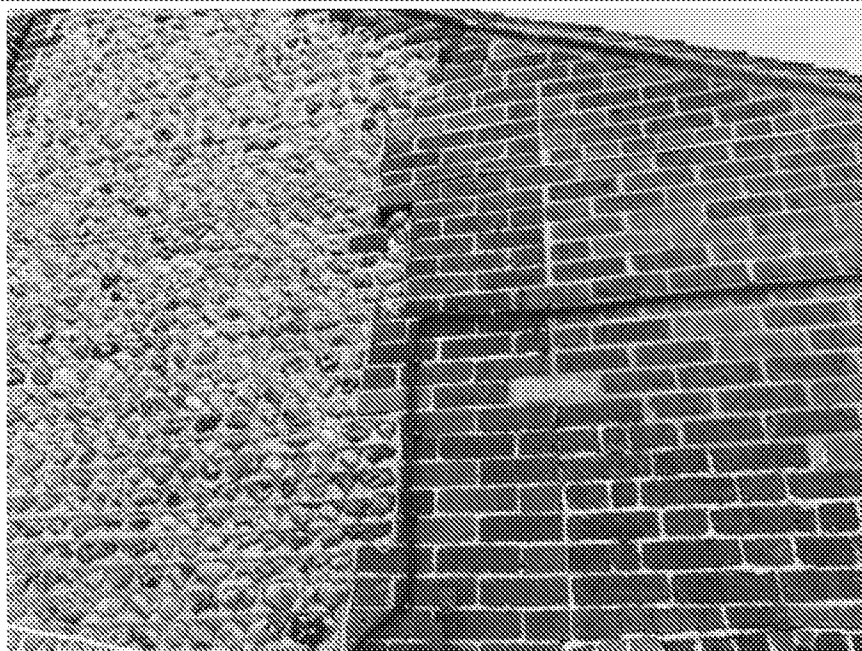
Building 4 – Side elevation to rear of building 3 showing cracking between flint and brickwork
