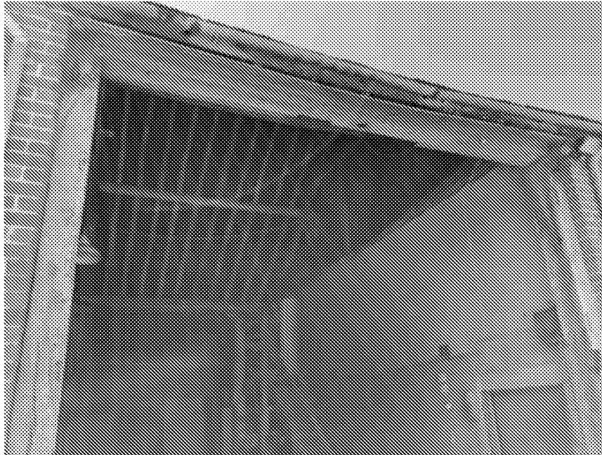
Building 4 – Sagging timber beam at eaves level of door opening
