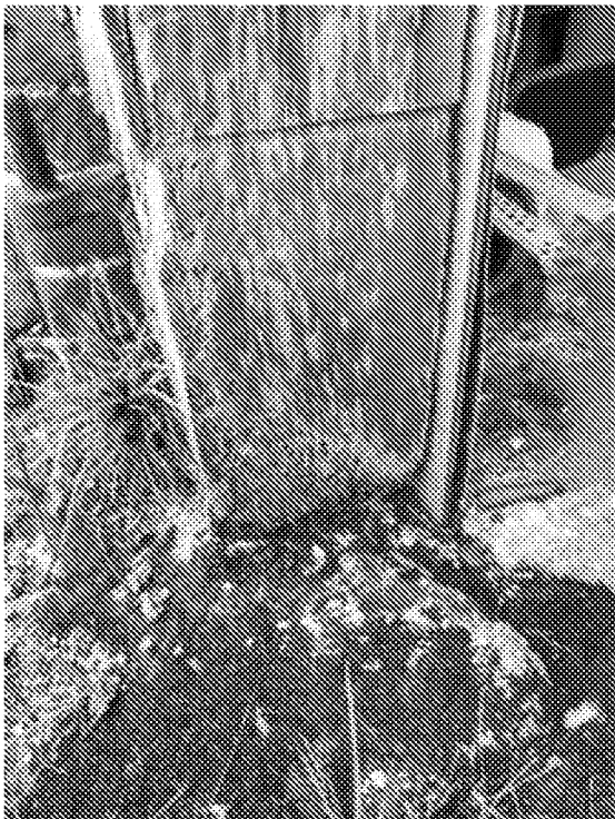
Building 4 – Rotten base of post to door opening
