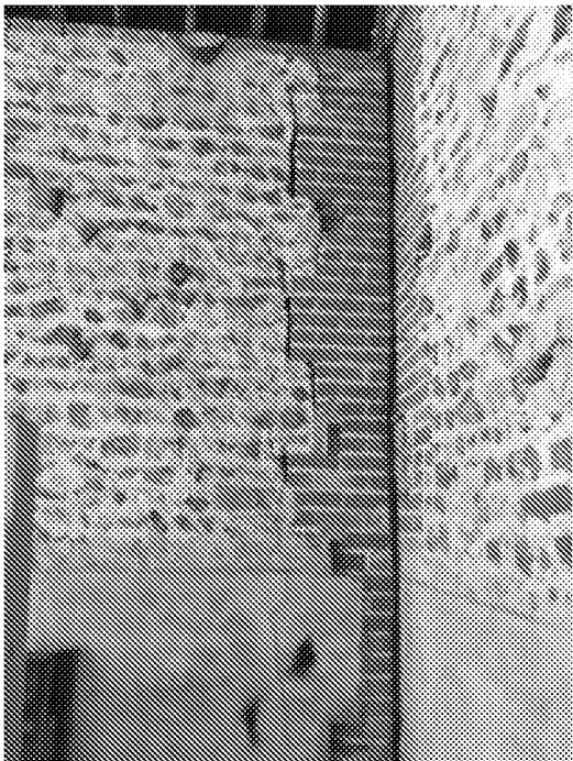
Building 4 – Typical vertical cracking between brickwork and flint
