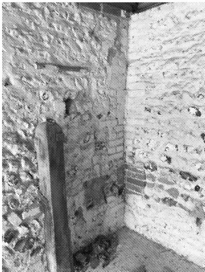
Building 3 – Cracking at internal return wall and rear wall
