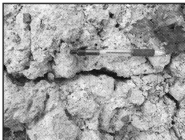
Plate 2: Example of soil shrinkage cracking
