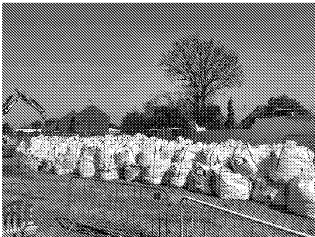
Figure 17: Double lined bags containing asbestos materials
