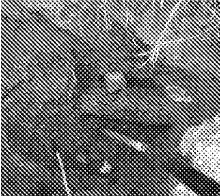
Figure 8: Soil is broken around the underground cable
