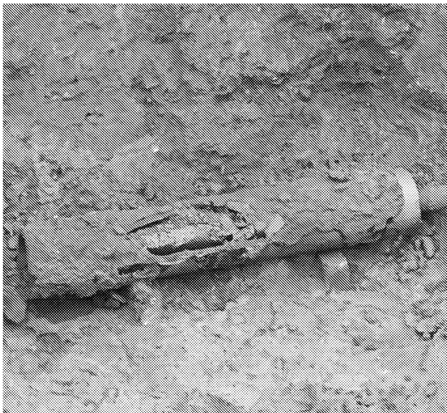
Figure 9: The cable is fully exposed
