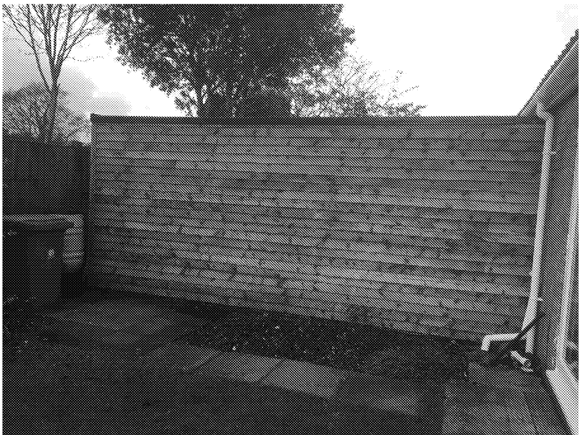
This is the new structure and it can be seen that this is on the boundary and encroaches in to the garden.
