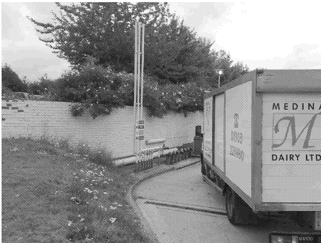
Photograph C –Tank vent stack and above ground off-set fill points
