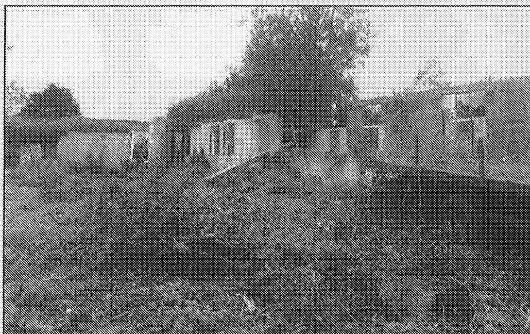
Figure 3: The western elevation of Building 1, showing the poor condition and missing roof over much of the building.
