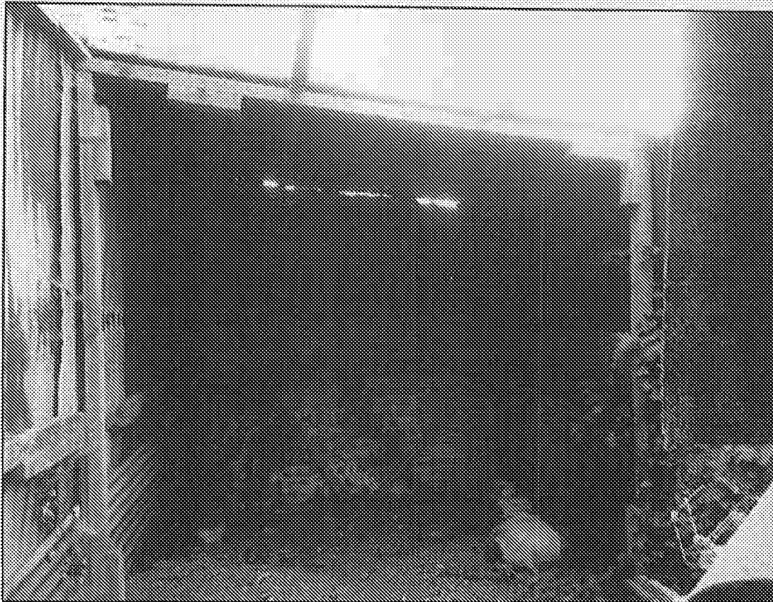
Figure 8: Showing the interior of Building 2 with gaps at the wall tops.
