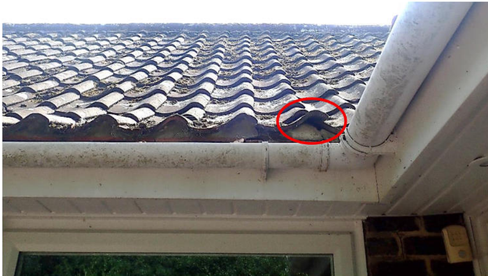
Fig. 4 – Tight fitting tiles at front (N) of property; gap where mortar has been lost
