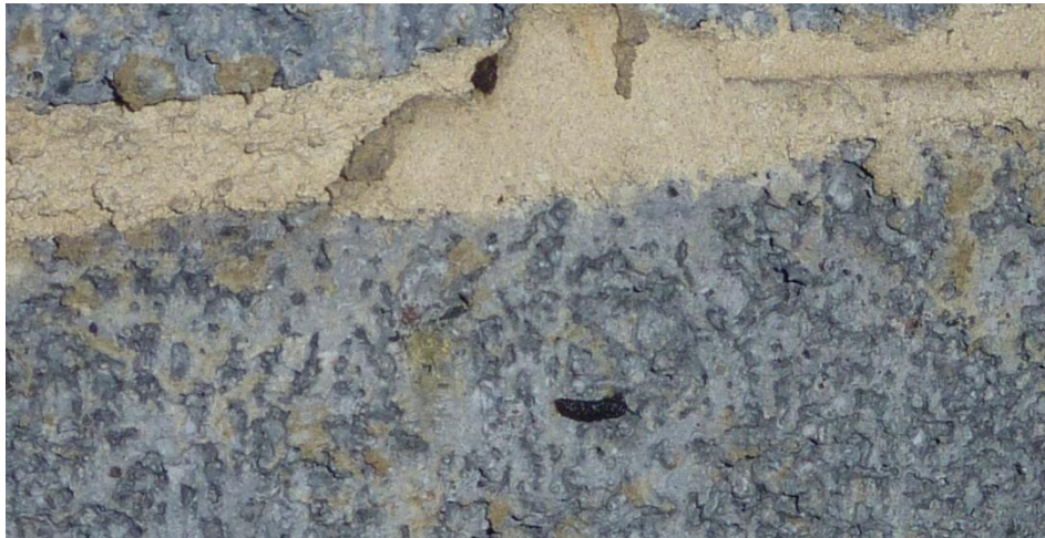
Fig. 11 – Small bat dropping, possibly from pipistrelle ( Pipistrellus sp.) on internal gable wall, E end
