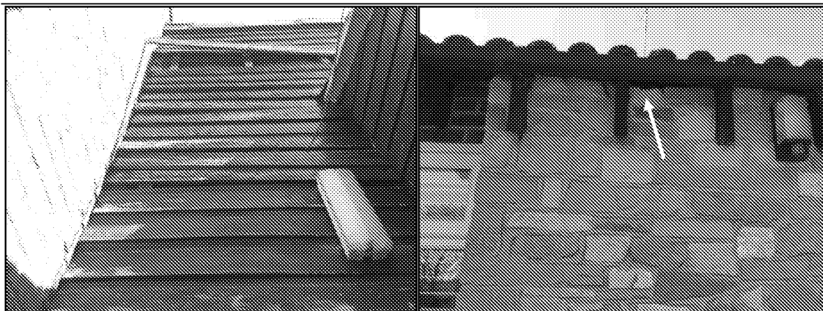
Photograph 13. Left image: gaps in unmaintained weatherboarding on the northern section of the house. Right image: gap in the mortar on the eastern face of the property (see white arrow).
