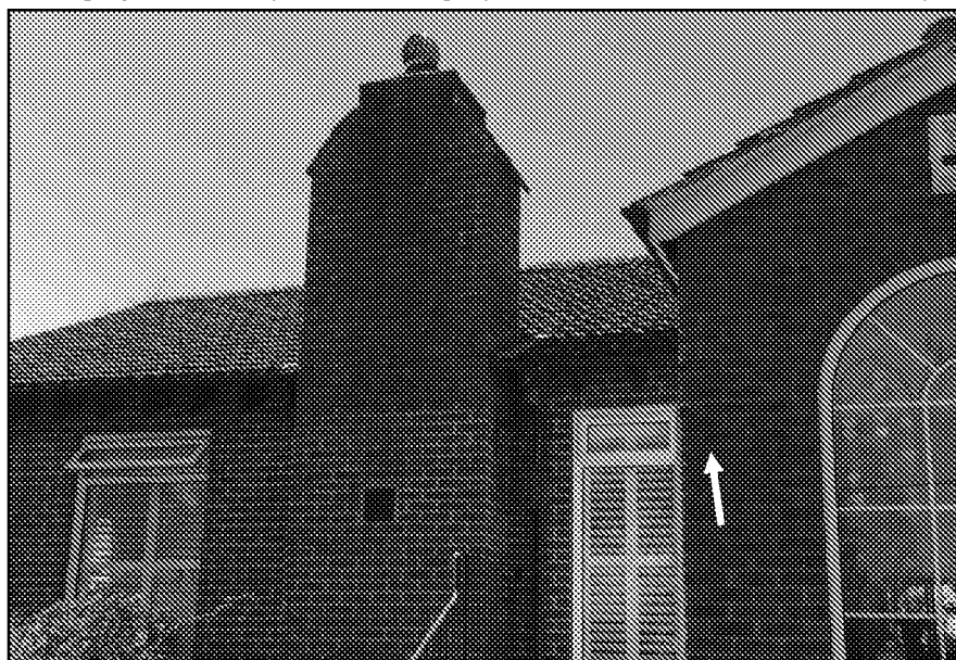
Photograph 15. A single raised tile east of the chimney on the eastern roof face of the property (white arrow).
