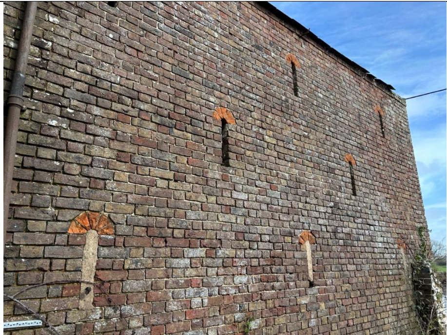
Photograph 13: Ventilation slits on B3 with some boarded on the outside
