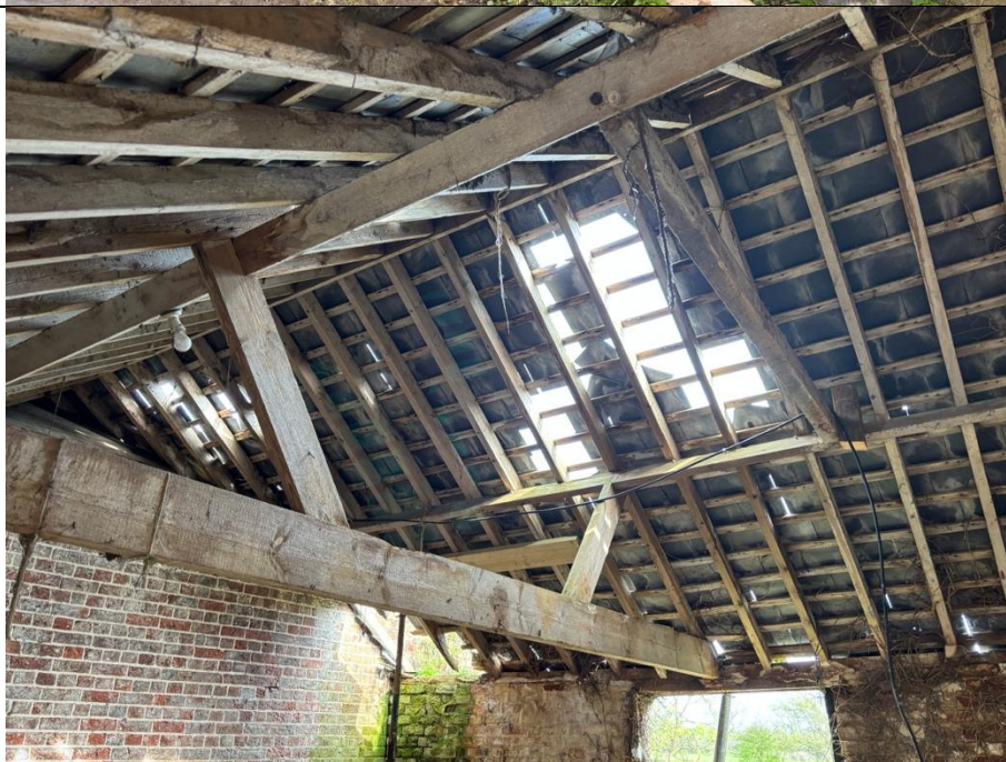
Photograph 24: Inside B8, no underlay for the roof, missing tiles lets light into the building
