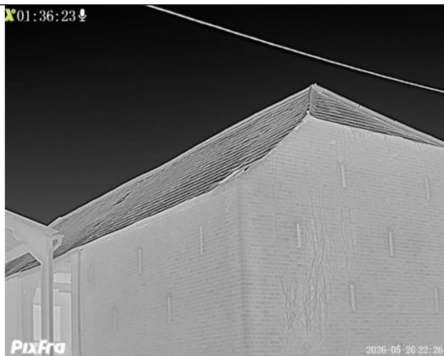
Figure 9: Screenshot of Thermal footage to the south-east of B3 on 20/05/26
