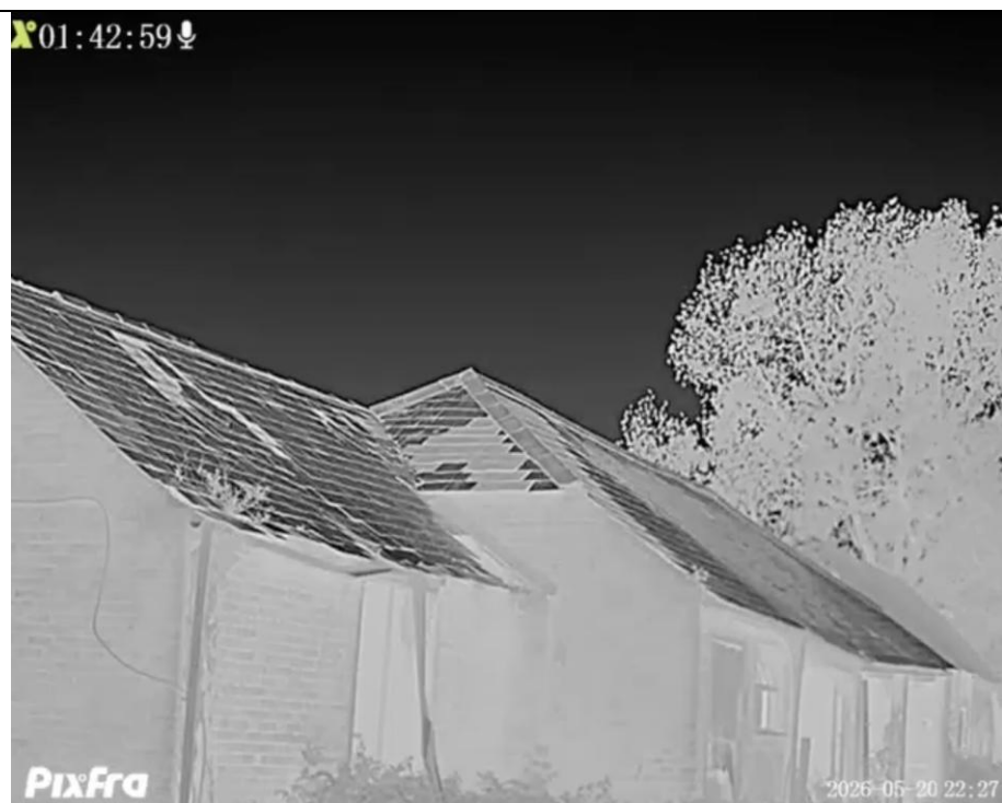
Figure 11: Screenshot of Thermal footage to the south-east of B8 on 20/05/26
