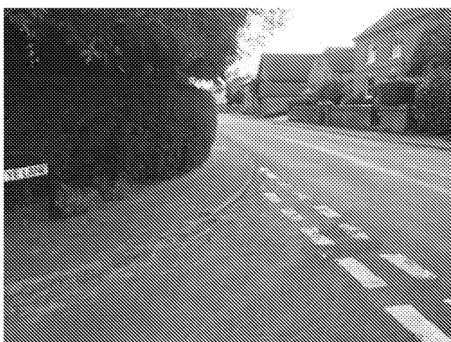
Figure 3: Worn carriageway markings.
