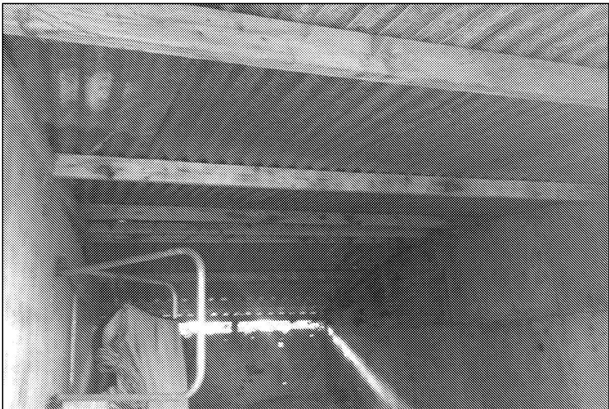
Figure 16. The corrugated roof and large gap within part of Stable Building 2.
