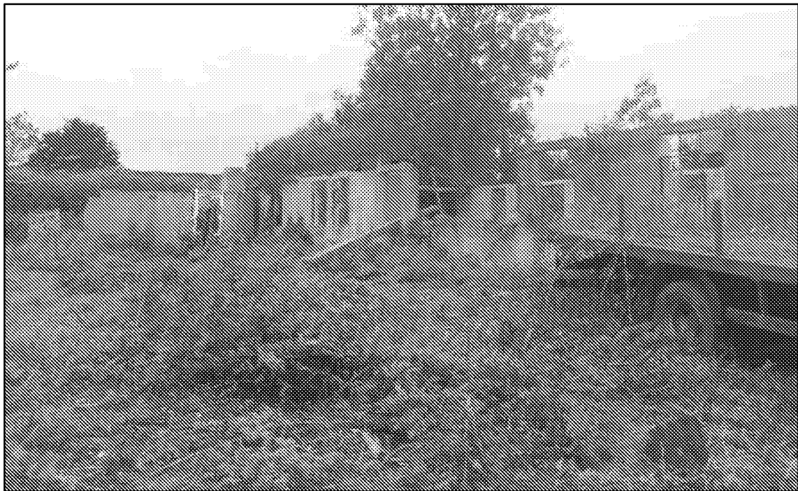
Figure 3: The western elevation of Building 1, showing the poor condition and missing roof over much of the building.
