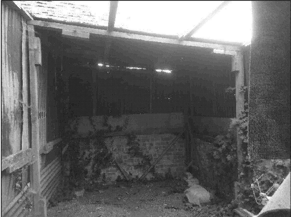
Figure 8: Showing the interior of Building 2 with gaps at the wall tops.
