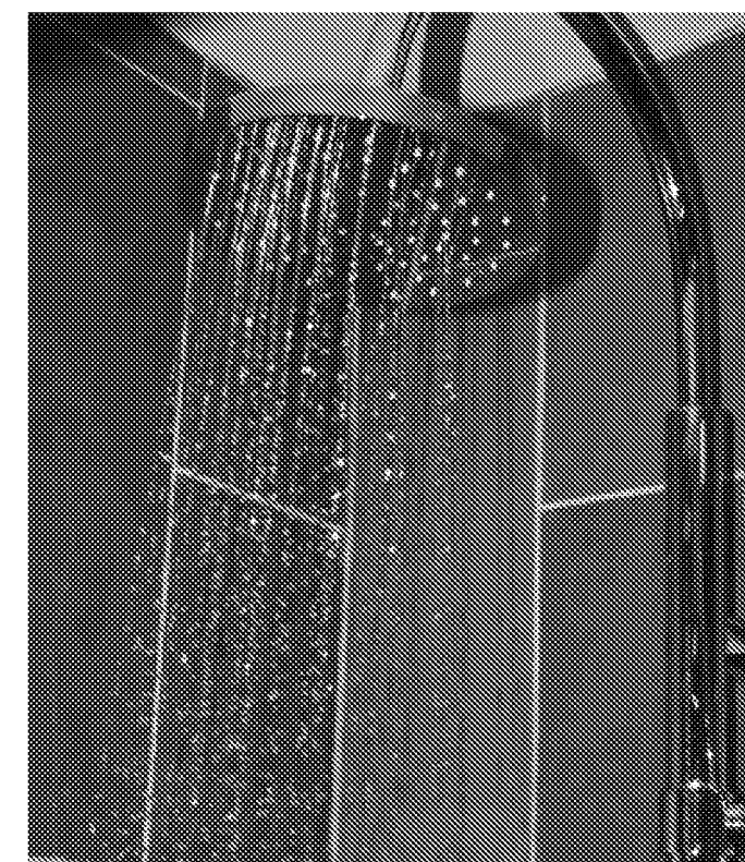
Low water usage fittings installed in all dwellings
