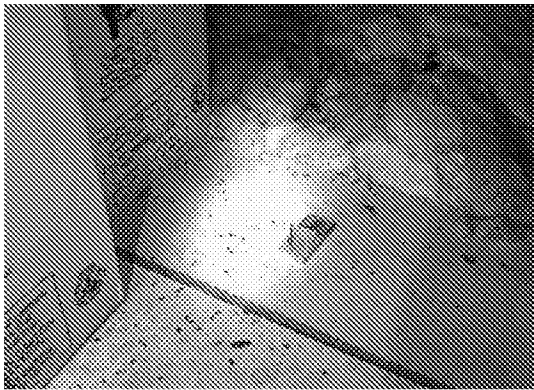
P9. Scattered bat droppings n roof space (from ESL 2020)
