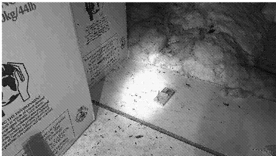
Numerous bat droppings in the loft of the house
