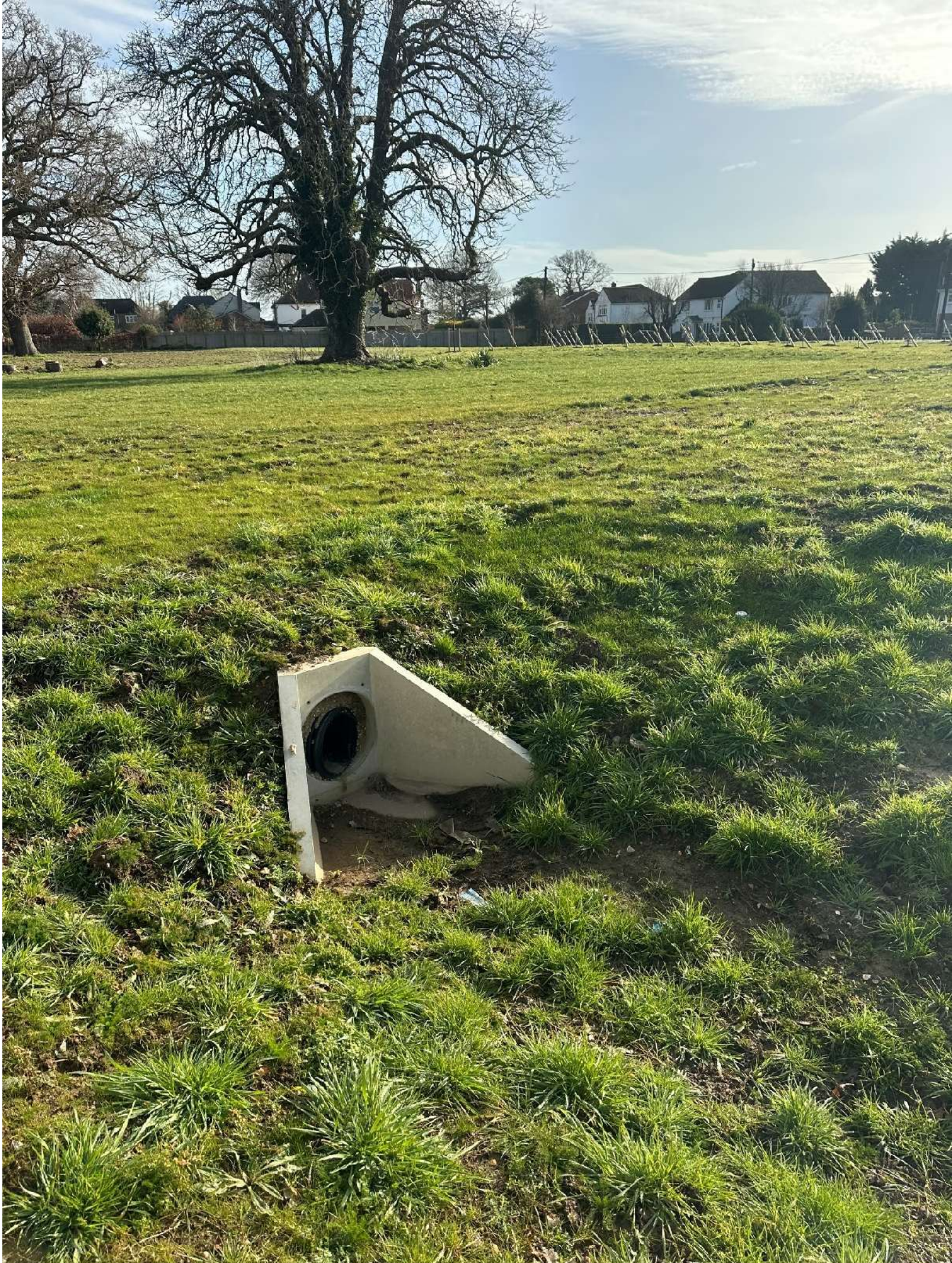
Head Wall 1G - 01 February 2023 - complete and functioning
