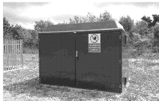
Customer Substation, Tavells Farm, Hampshire
