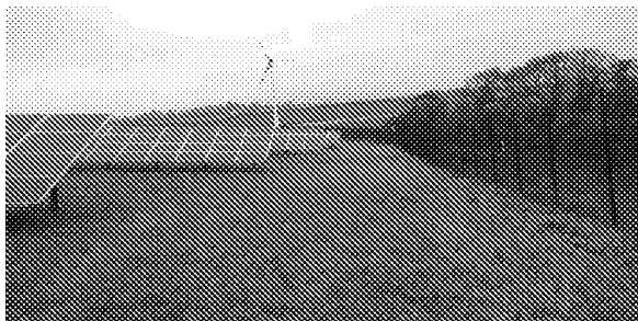
Ninnis Solar Farm, Cornwall
