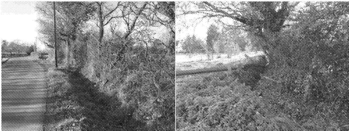
Figures 2 & 3: Open ditches in the route of the footway links.
