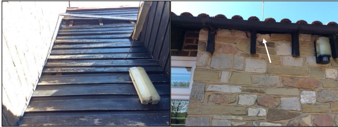
Photograph 13. Left image: gaps in unmaintained weatherboarding on the northern section of the house. Right image: gap in the mortar on the eastern face of the property (see white arrow).
