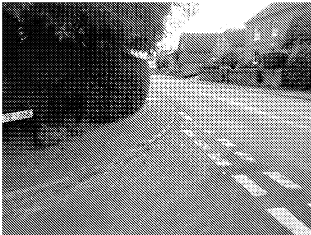
Figure 3: Worn carriageway markings.
