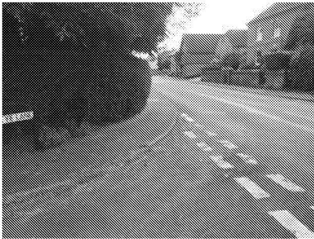
Figure 3: Worn carriageway markings.
