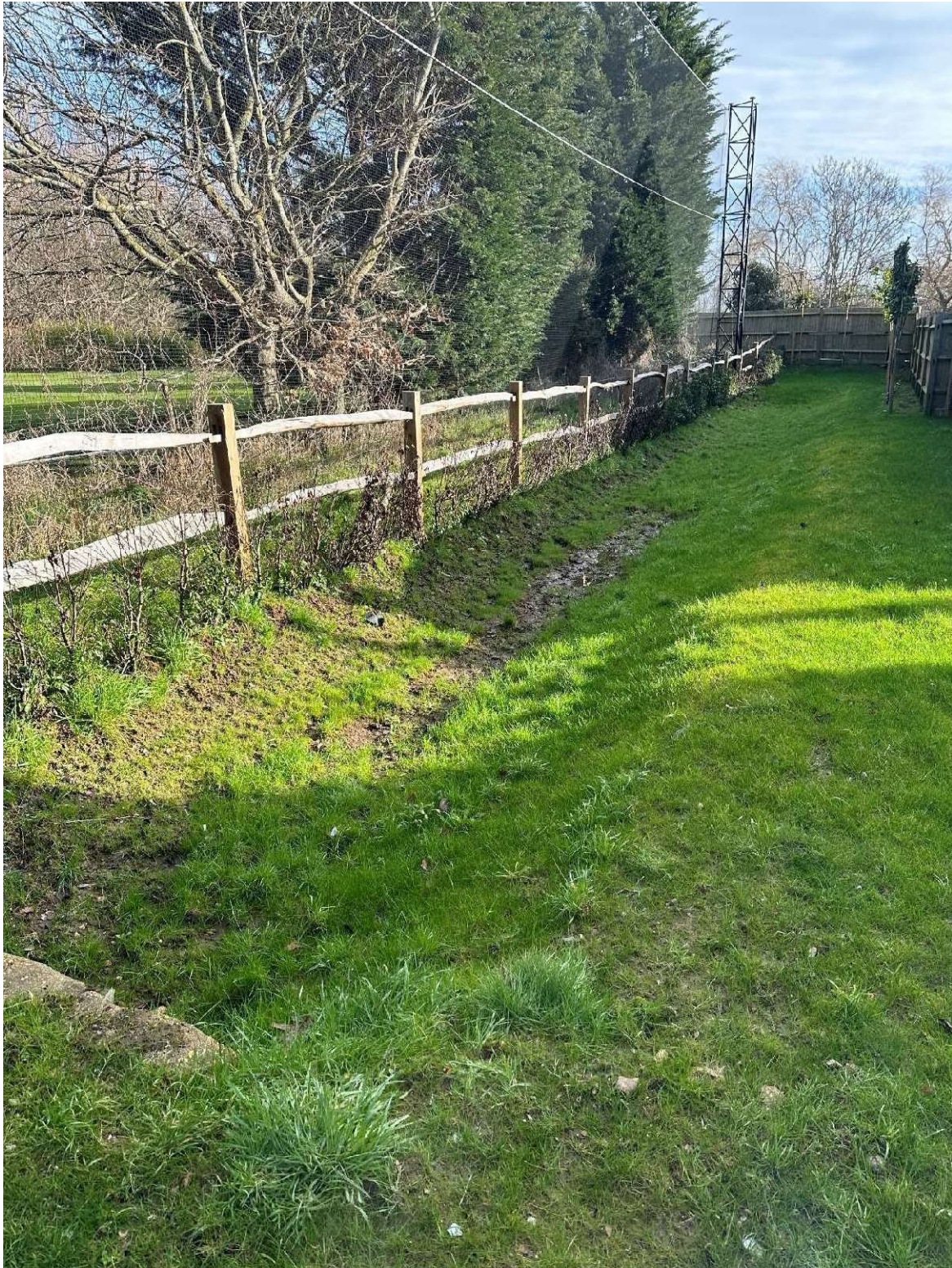
Swale D - 01 February 2023 - complete and functioning
