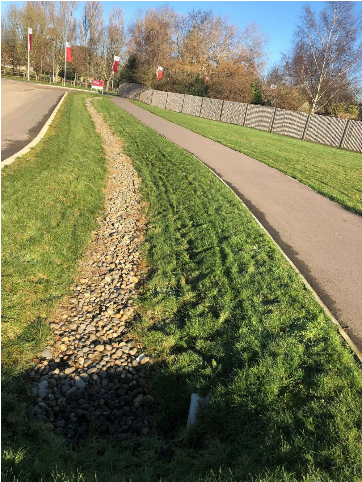
Swale E - 17 January 2022 - complete and functioning
