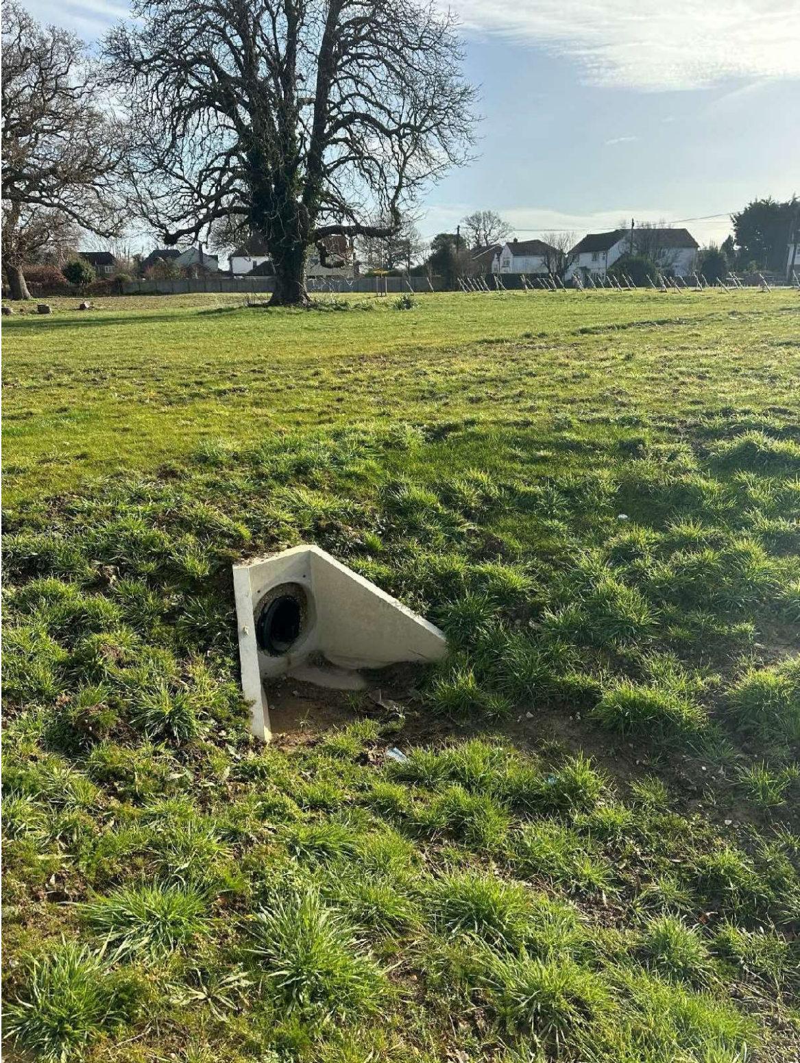
Head Wall 1G - 01 February 2023 - complete and functioning
