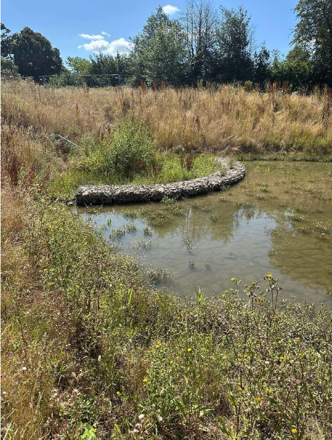
Western Basin – 16 th July 2025 - complete and functioning
