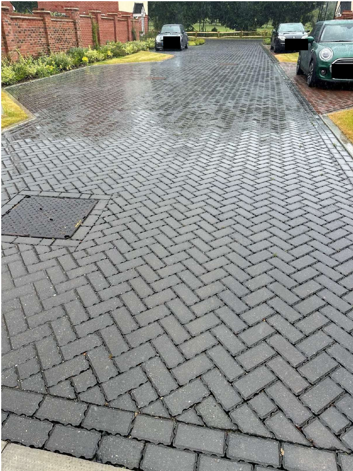
Permeable Pavement 2A - 9 July 2024 - complete and functioning
