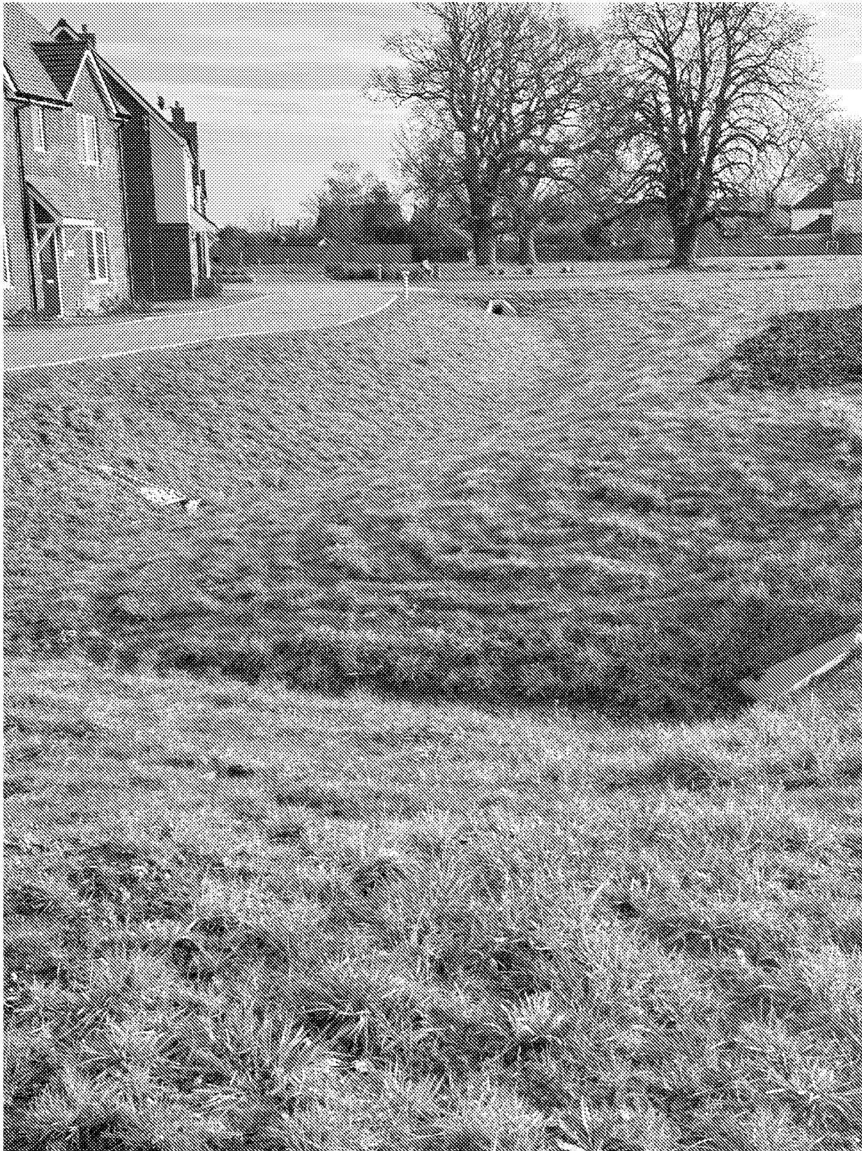
Swale 1H - 01 February 2023 - complete and functioning
