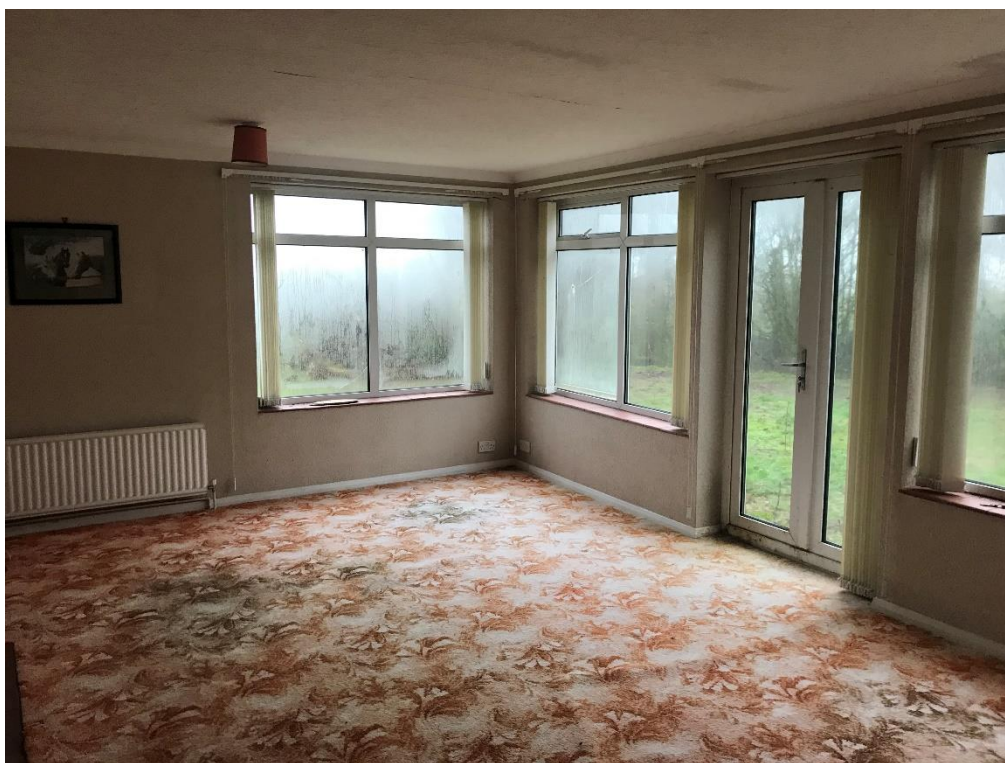
Plate XII : Ground floor rear flat roofed area – Damp ingress to ceiling and failed glazing
