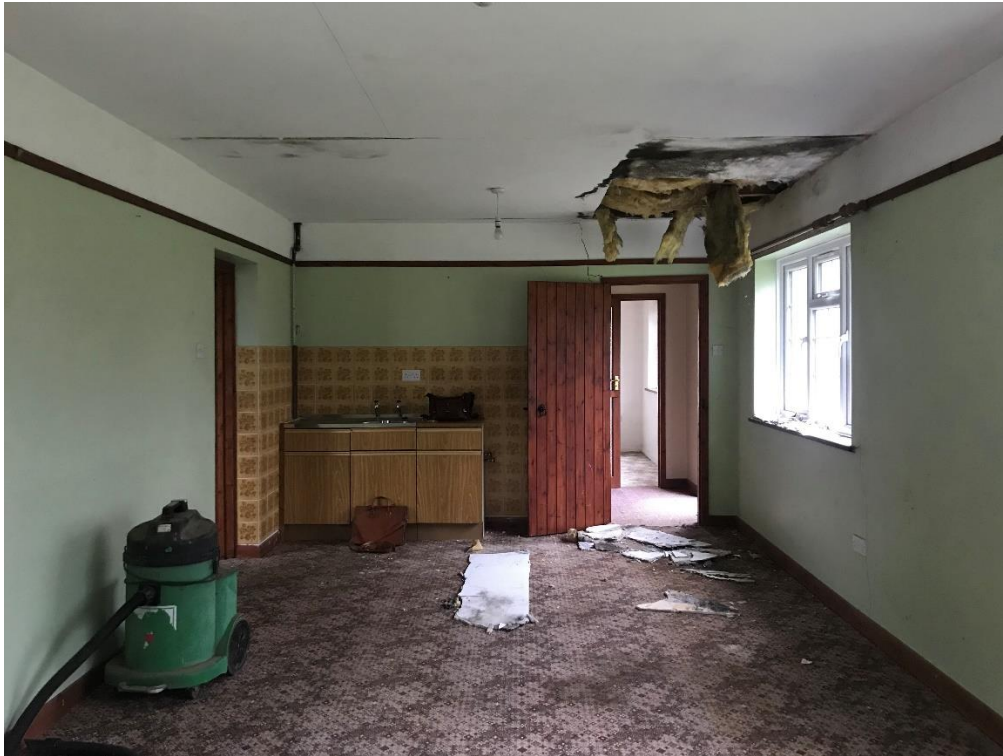
Plate VIII : Ground floor dining room – damaged ceiling with water ingress to the failing roof covering
