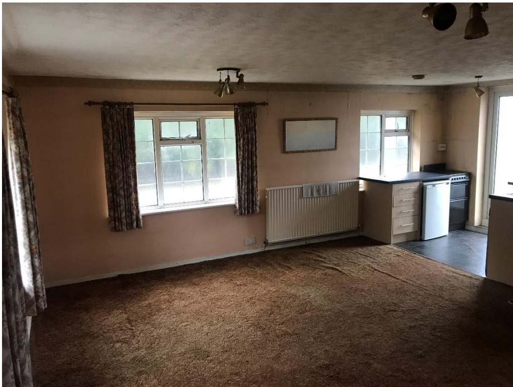
Plate XV : First floor north bedroom – Mould growth and worn fittings
