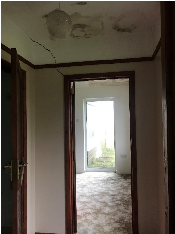
Plate XI : Rear ground floor - Structural cracking and water damage
