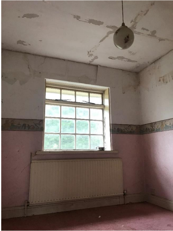
Plate XIV : First floor – front bedroom with signs of rainwater ingress.
