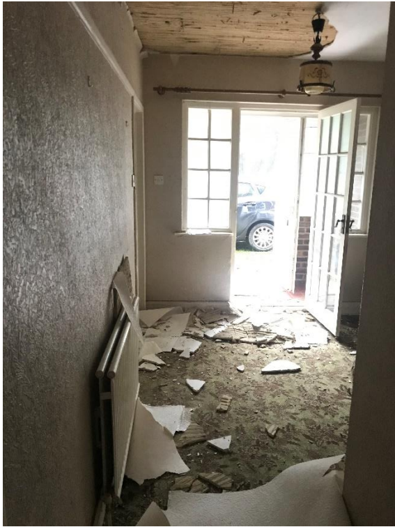
Plate VI : Ground floor entrance hall – damaged ceiling
