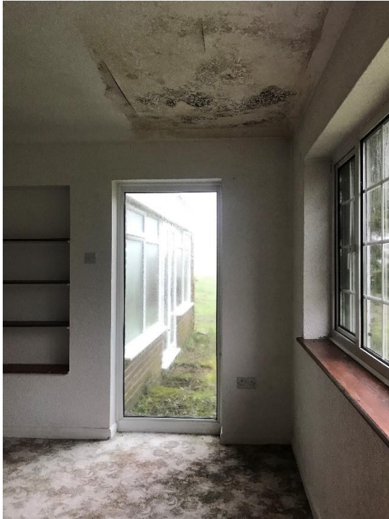
Plate X : Ground floor rear reception room – Further water ingress damage to ceilings
