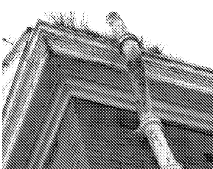
FIG . 35 - PBA PHOTO - BLOCKED GUTTER
