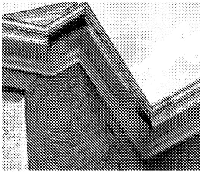
FIG . 38 - PBA PHOTO - CORNICE SHOWING SIGNIFICANT DECAY
