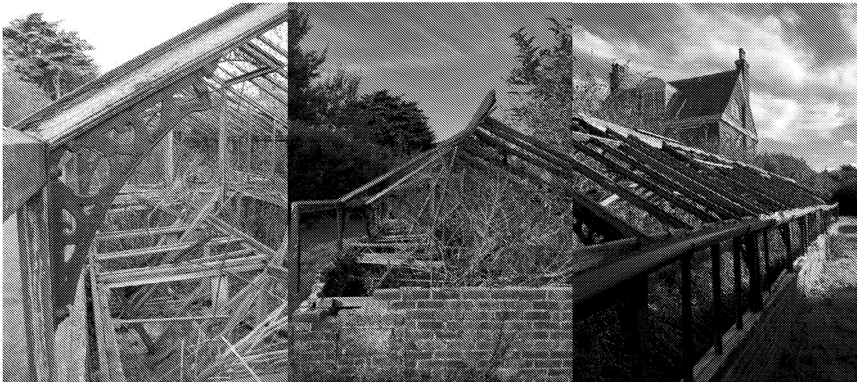
FIG . 29 - PBA PHOTO MONTAGE - DERELICT GLASSHOUSE
