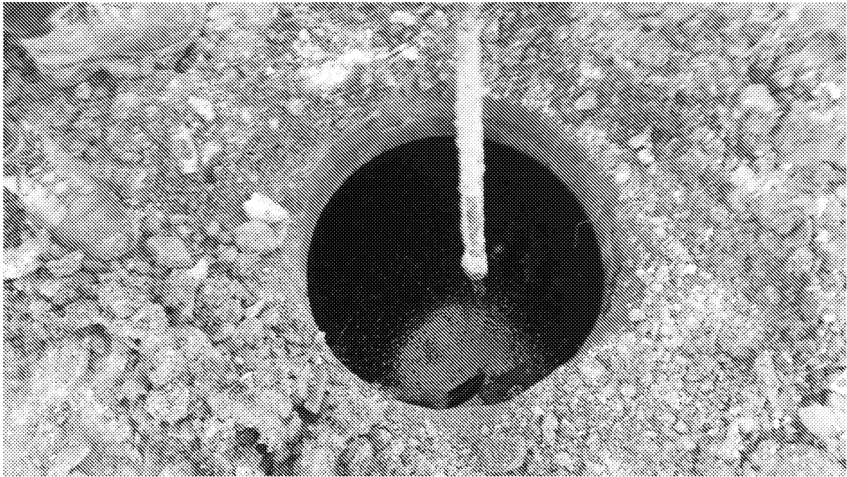
Figure 4 - Former soakaway filled with impacted material (Southern Source)
