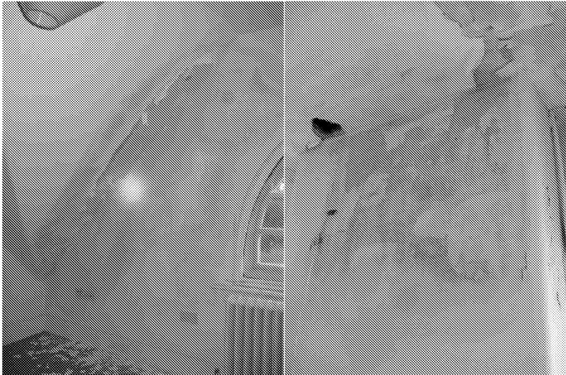
FIG . 33 - PBA PHOTO MONTAGE - DAMP AT SECOND FLOOR LEVEL
