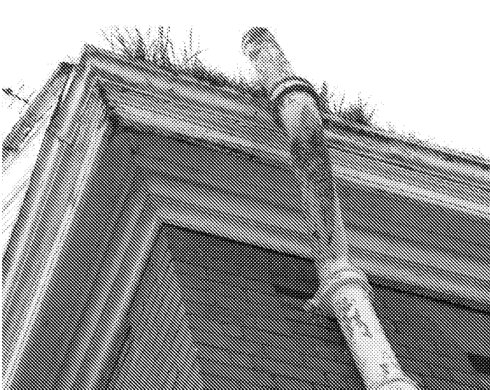
FIG . 35 - PBA PHOTO - BLOCKED GUTTER
