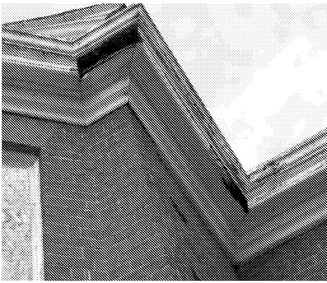
FIG . 38 - PBA PHOTO - CORNICE SHOWING SIGNIFICANT DECAY
